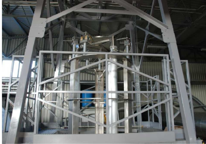
Figure 11.5: The monolithic IP prototype installed in SAFE.
