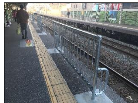
[ホーム固定柵(笹原駅)]
