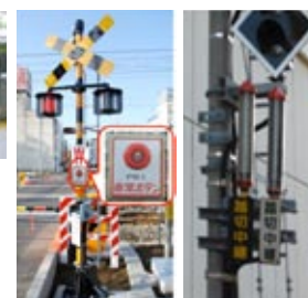
(Emergency button) (Obstruction warning signal) Level crossing warning system
