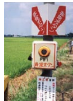
Level crossing alarm system
