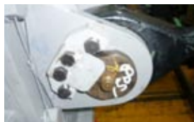
Metal fittings to prevent unfastening of the pins that support reduction gears
