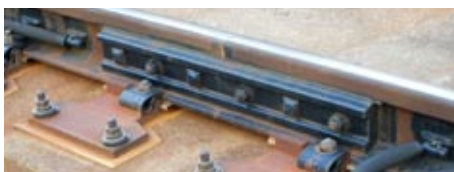
Before improving glued insulated joints
