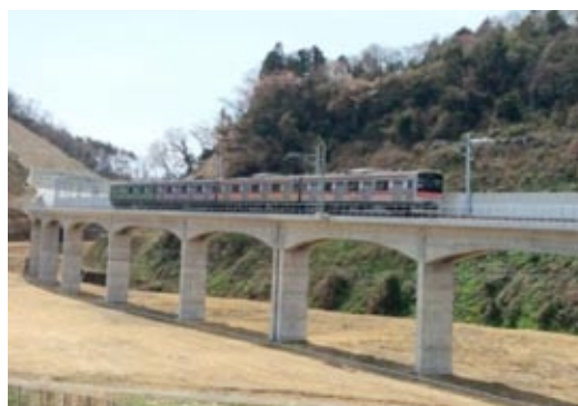
Senseki Line (between Nobiru and Rikuzenono)
