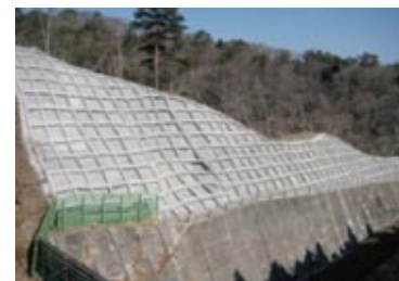
Natural slope protection (spray frame work)
