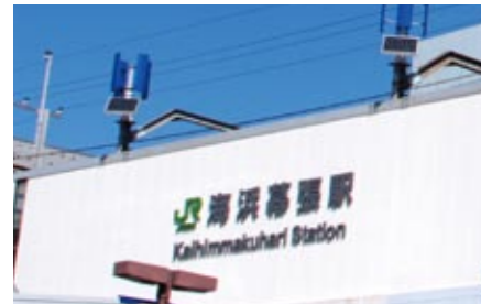
Small-sized wind power generation facility installed at Kaihinhakuhari Station
