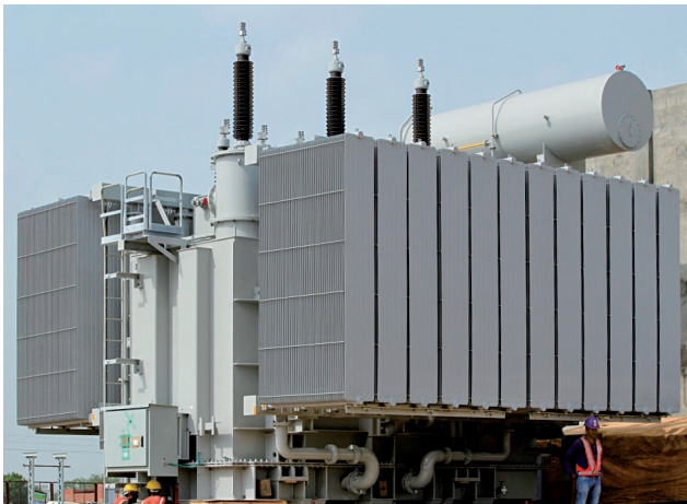
現地に据え付けられたスコット変圧器 Scott connected transformer installed on-site in dedicated freight corridor, India
