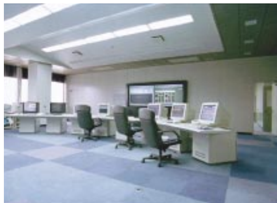
“中央受配水場”監視室 Operation room of Izumi City “Tyuujuhaisuijo”
