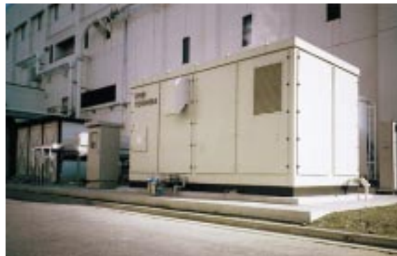
汚泥消化ガス燃料電池発電設備 Fuel cell power plant running on anaerobic digester gas
