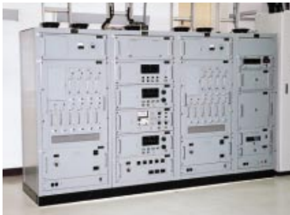
距離測定装置 Distance measuring equipment
