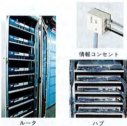
LAN システム構成機器 LAN system configuration equipment
