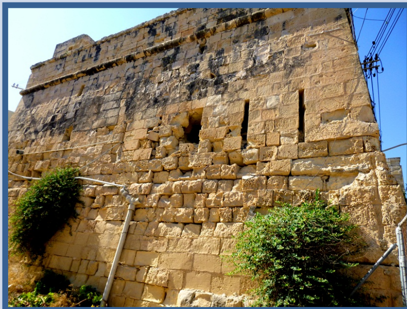
The southern façade: in need of restoration
