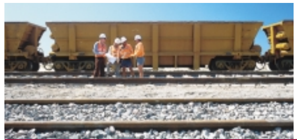
Continuous maintenance and on-going track upgrades enhance the safety of our rail network.
