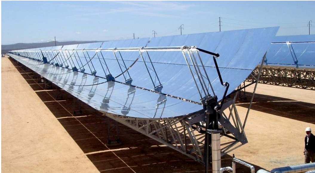
The core of the parabolic trough plant: the solar field with the solar collectors and the absorber tube (here: Solar Millennium Demonstration project at a power plant in California)
