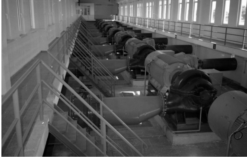
Figure - 6: Pumping Station ( Ülger, 2004 )
