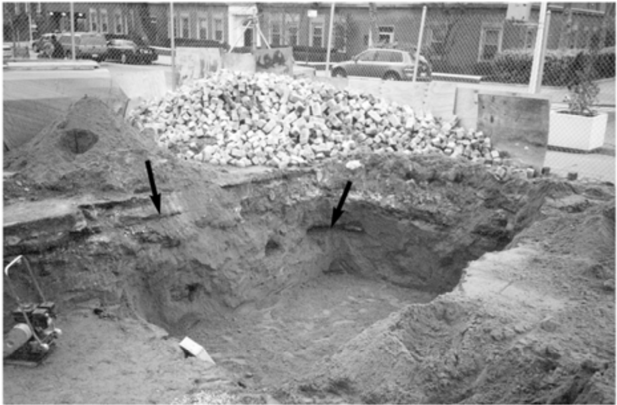
20 Pit 1 (north of West Pier) at end of excavation looking northwest. Note Belgian block removed from pit and rubble above a buried asphalt layer (left arrow). Also, chunks of asphalt (right arrow) in fill. (Spritzer March 9, 2004)
