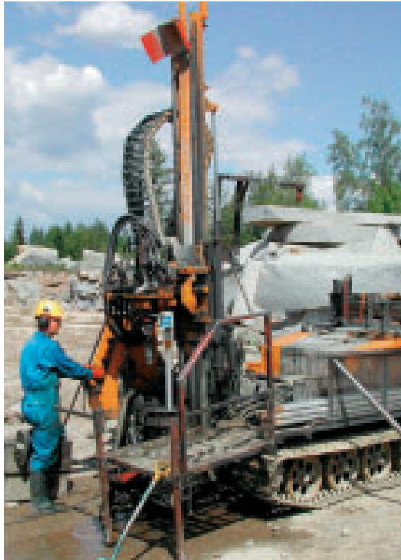
Diamond drilling in progress as part of an investigation of a natural stone site in Pirkanmaa. Photo: Paavo Härnä
