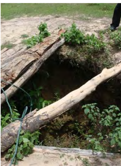
Figure 18 - Unprotected well used by families
