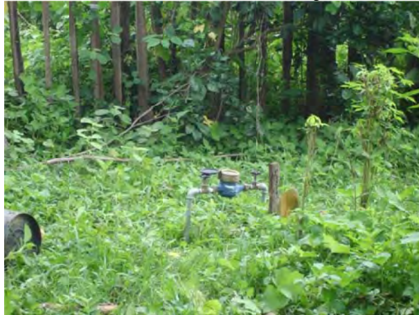
Figure 34 - Household meter with no protection
