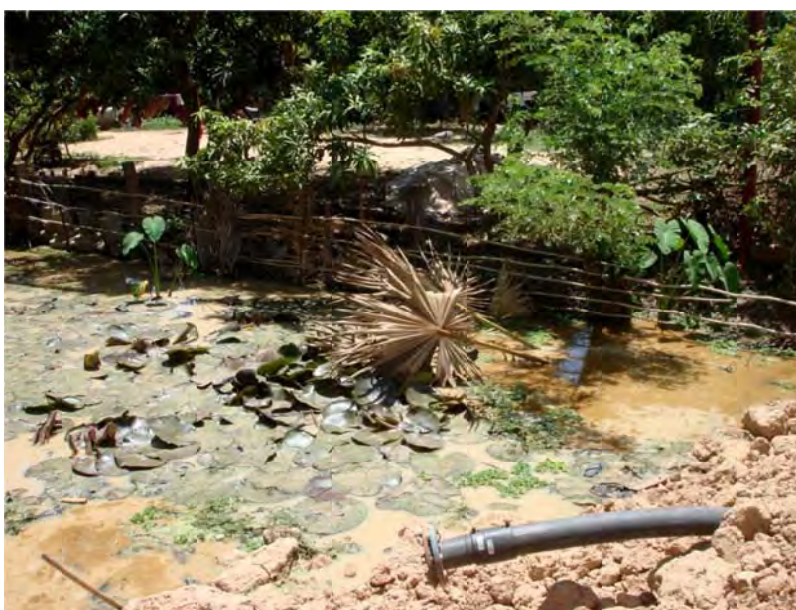
Figure 13 - Section of the system where the distribution line ends. Expansion is needed.
