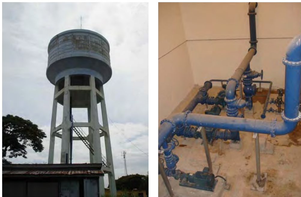
Figure 17 - Reservoir and pumping station for the system
