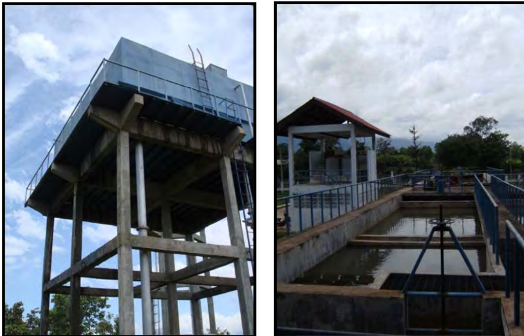
Figure 35 - Water treatment plant and leakages in reservoir (constructed in 2006)
