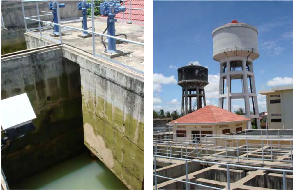
Figure 8 - Kampong Thom water treatment plant and elevated tanks
