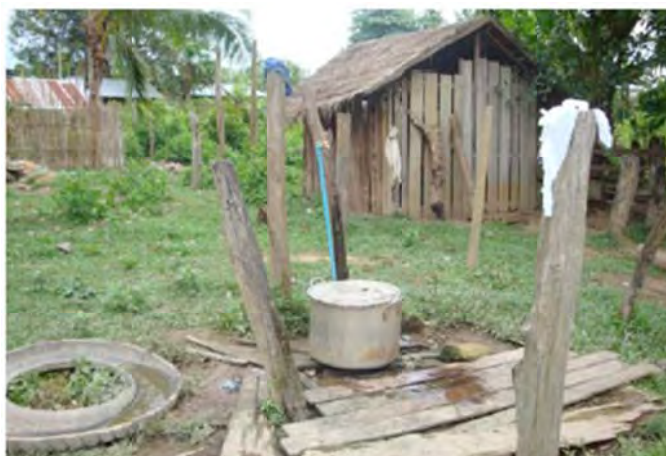
Figure 25 - Shared connection to the water network in a poor area
