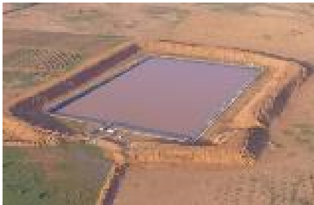
Earth pan with dam liners at Ramad and Galool. Photo credit: [REDACTED]/GEEL
