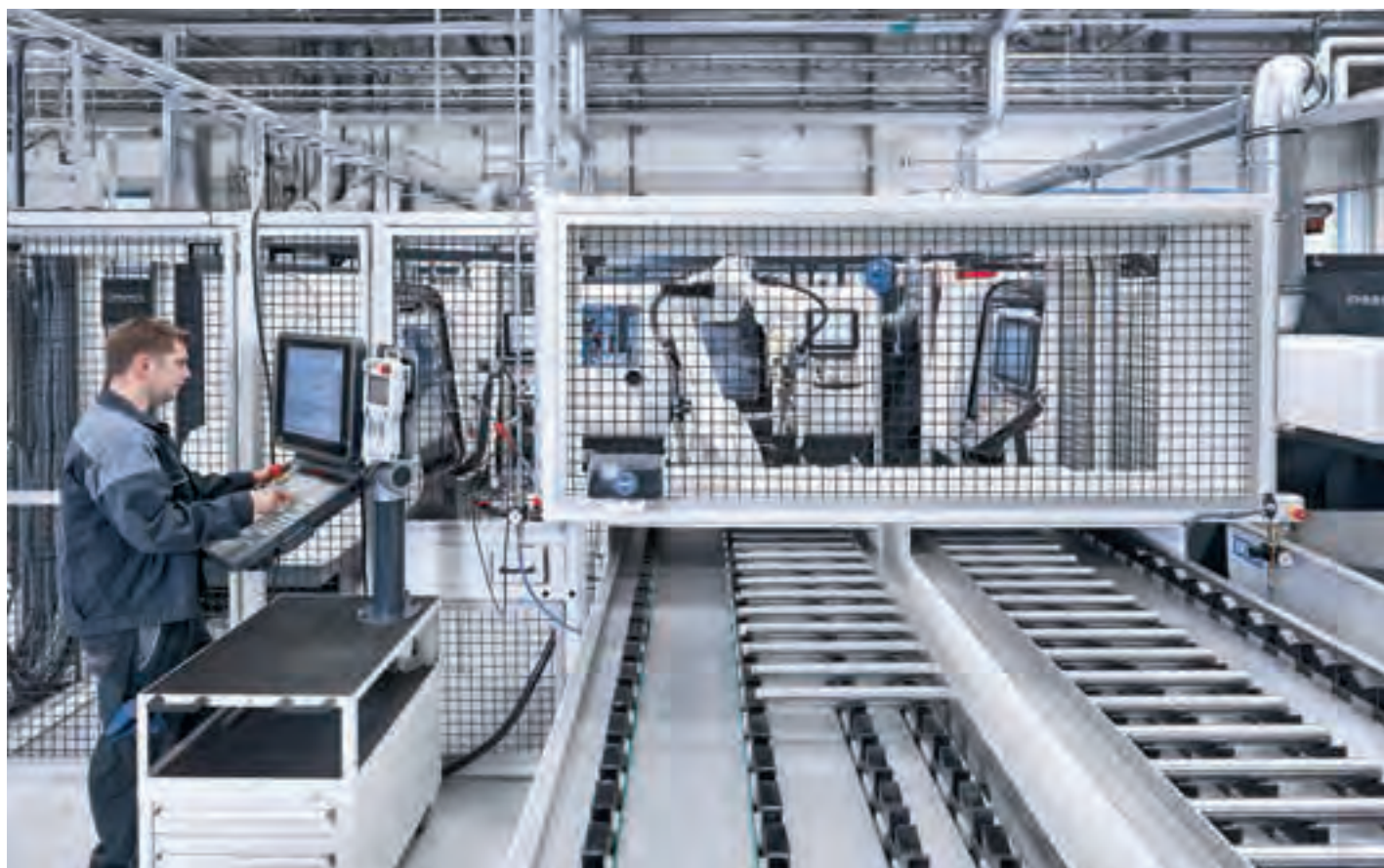
Two conveyors handle loading and unloading of the production cell. All other processes, including integral measuring of the workpieces, are carried out completely automatically.
