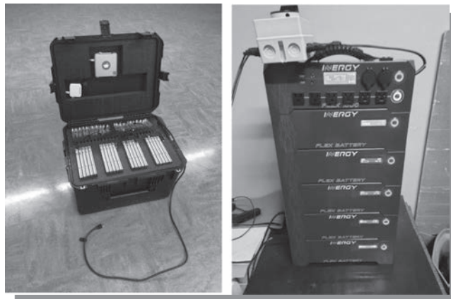
SmartBox and Solar Power system installed in the village of Empash
