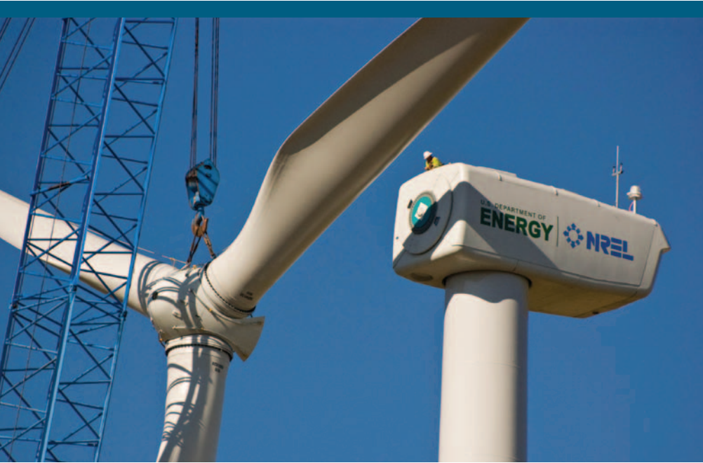
Blue skies and calm conditions contributed to a smooth installation of the DOE 1.5 megawatt wind turbine at the National Wind Technology Center.
