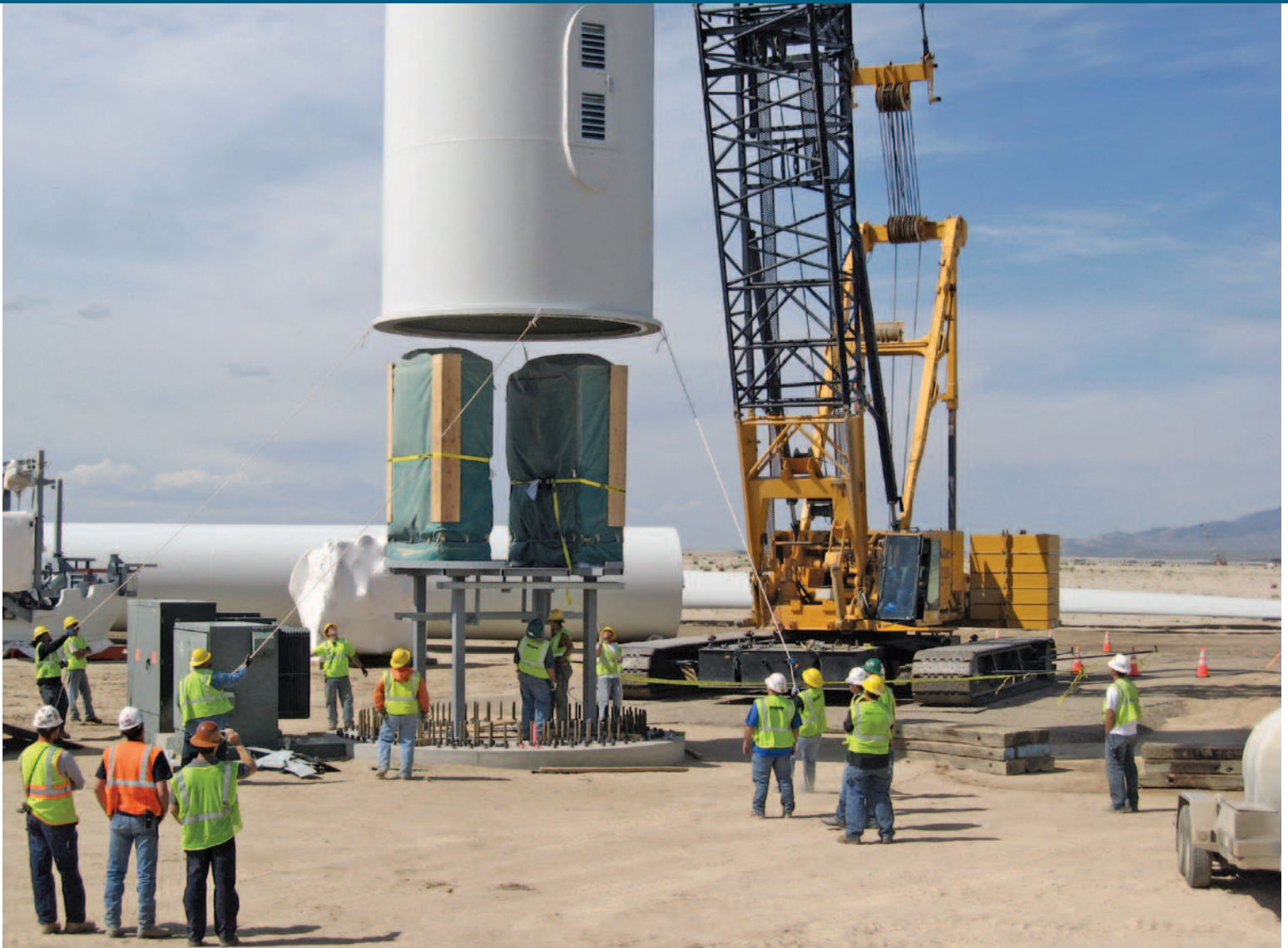
Construction workers in Milford, Utah, lower the first section of a tower for a multimegawatt wind turbine.
