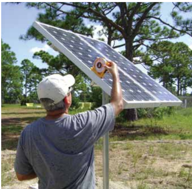
A worker with Geosyntec Consultants Inc. checks the orientation of a solar panel with an inclinometer at Kennedy Space Center. The solar panel powers a recirculation system that is removing contamination from the groundwater at this site.
