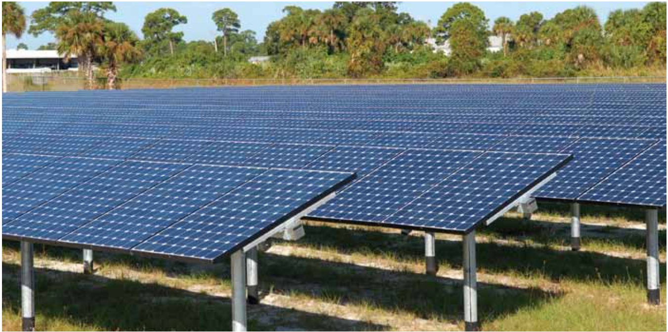
NASA's first large-scale power generation facility opens at Kennedy Space Center in November 2009. The one-megawatt facility features a fixed-tilt, ground-mounted solar power system that will provide energy to the center.
