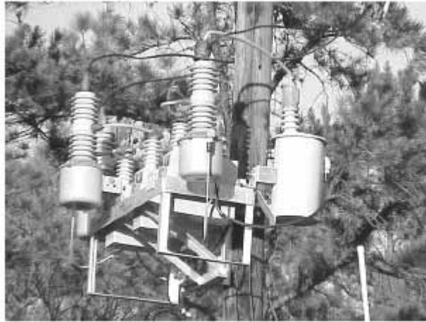
Fig. 2. Switched capacitor banks improve voltage control and reduce system losses. (Note the white radio antenna at lower right for status monitoring by SCADA.)
