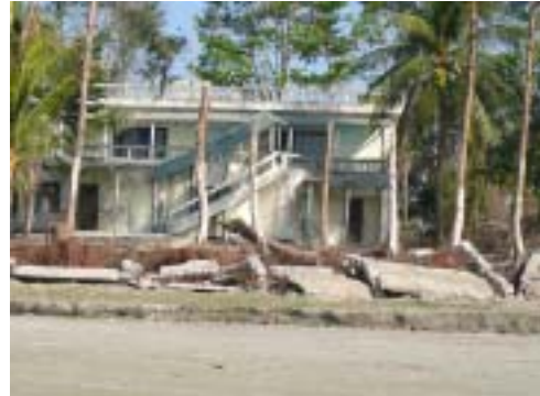
Fig.4 Damaged building of resort hotel in the Kuwakata coast
