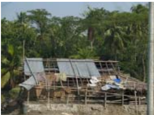
Fig.3 Damaged house in Sharankhola
