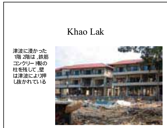
Photo. 6 Tsunami attacking three stories concrete made hotel at Khao Lak, Thailand.
