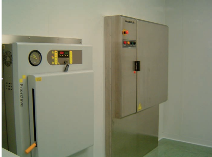
FIG. 3.5. Steam sterilizer and dry heat oven installation in a kit production facility (source: Monrol A.S.).
