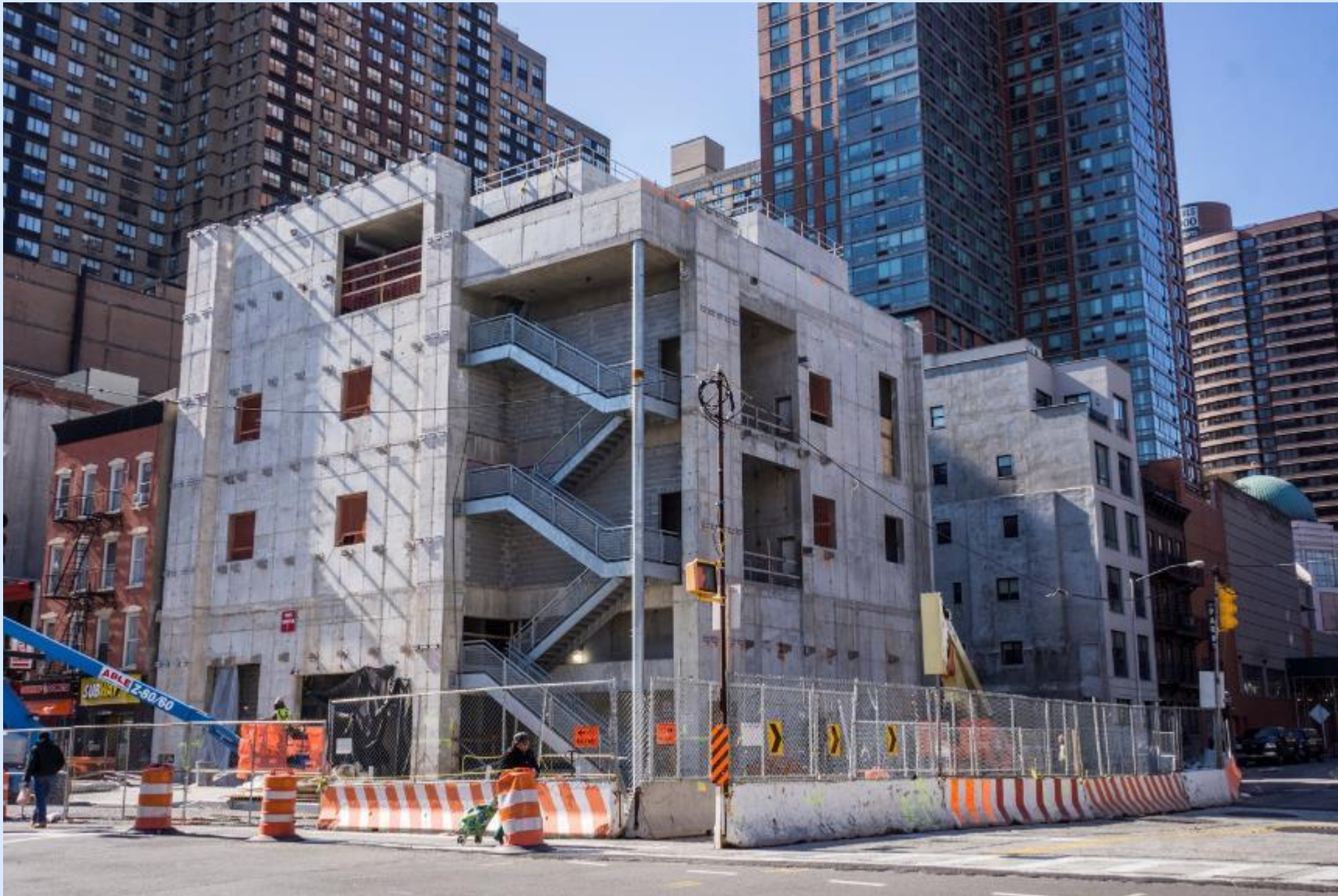
Ancillary 2 – Stairs with railing installed and clips for granite façade Southwest corner of 97 th Street & 2 nd Avenue
