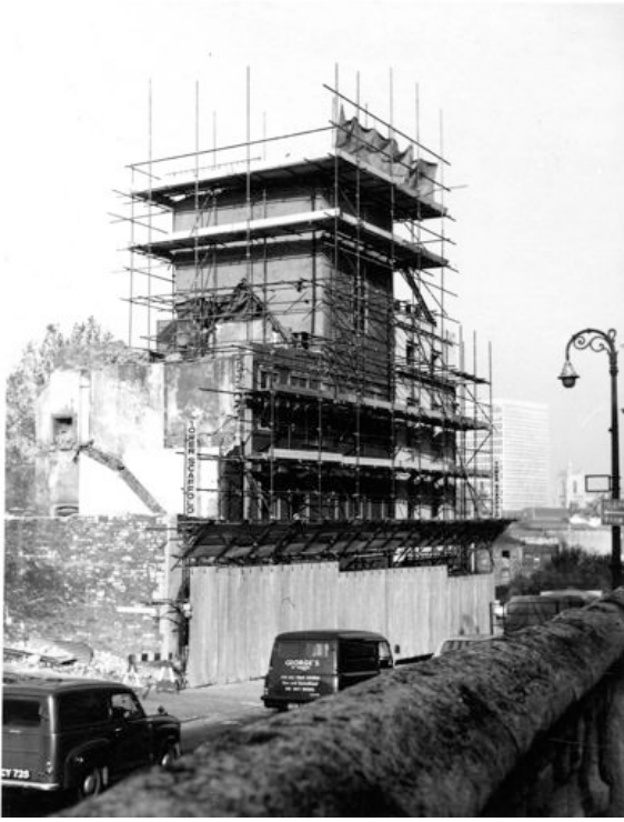
Ap. 03. The old shot tower in Redcliff Hill shrouded in scaffolding prior its demolition. November 1968.
