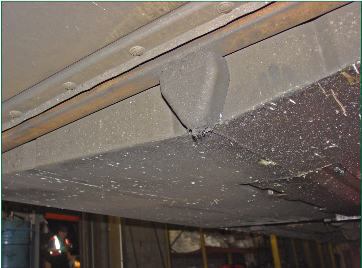
Figure 11: Plastic cover over fuel tank 'dead-space' drain valve
