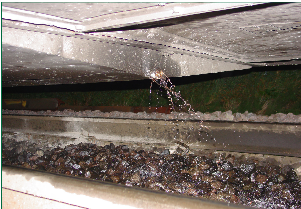
Figure 12: Fuel leaking from a damaged fuel tank 'dead-space' drain valve
