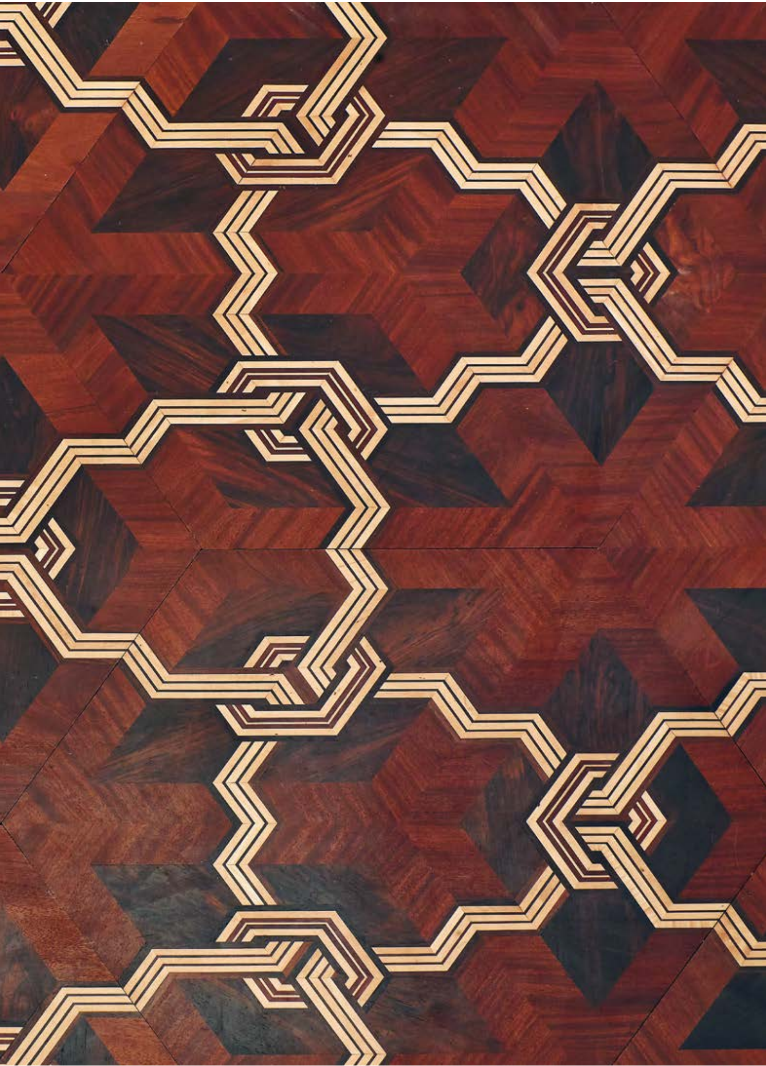
Detail of the inlaid parquet floor of the Square Room on the second floor piano nobile of the Liechtenstein City Palace, executed by Michael Thonet
