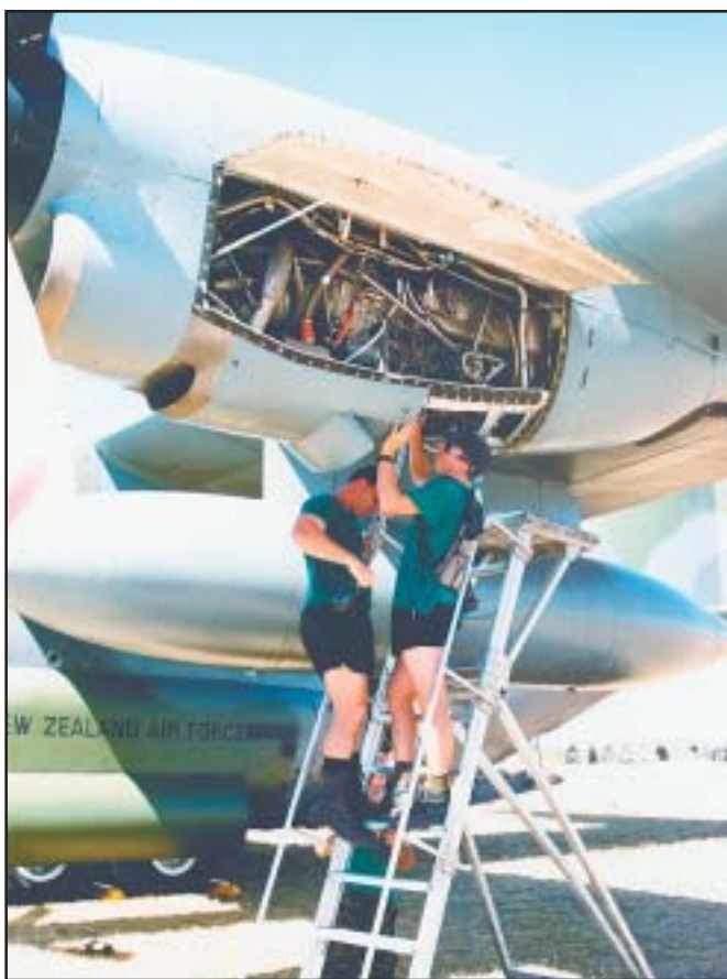
Left: Generally the T56 series engine has proven reliable in service world-wide although the RNZAF is fully equipped for an in field engine change if necessary.
