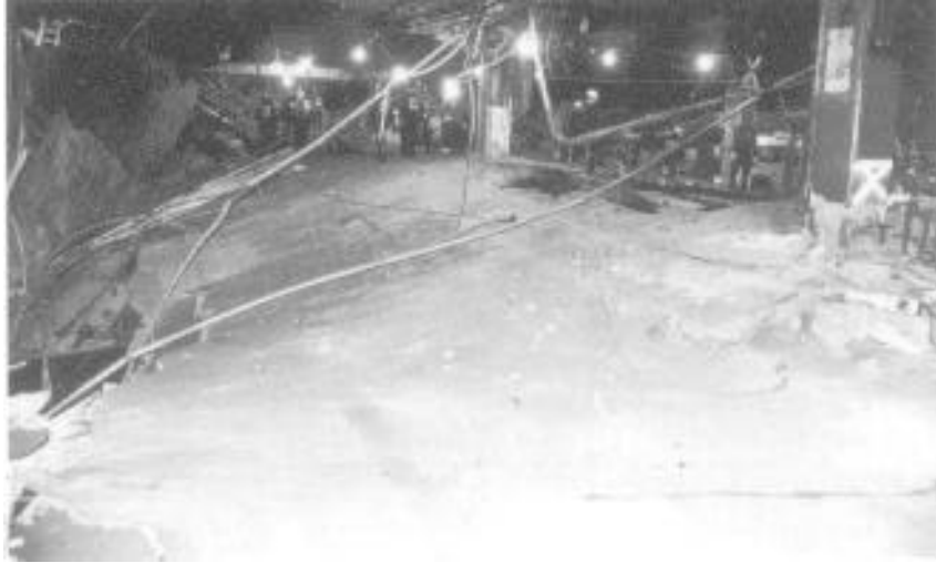
The sloping, hanging steel-reinforced concrete floor at the perimeter of the crater was a major hazard for units operating on the crater fire, particularly in the heavy smoke condition. (Photo by FDNY Photo Unit.)
