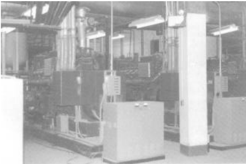
Emergency generators on the B-6 level. Cooling water lines for these units were ruptured by the blast, shutting down all emergency power. (Photo courtesy of Port Authority Risk Management.)
