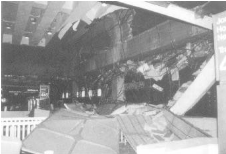
The explosion collapsed a portion of ceiling on the B-5 level onto a PATH train concourse. (Photos courtesy of Port Authority Risk Management.)
