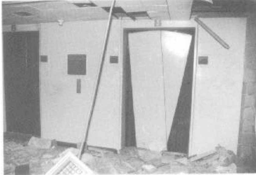
Damaged elevator doors and enclosures on the B-2 level presented a vertical channel for smoke spread into Tower 1. (Photo courtesy of Port Authority Risk Management.)
