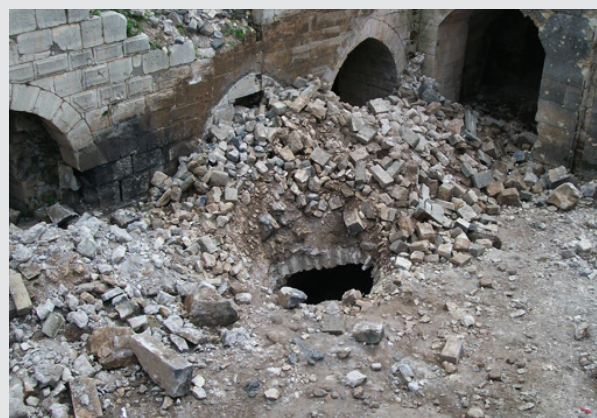
Image of the inner courtyard where the stairs have completely collapsed/Photo: DGAM, 03 July 2014
