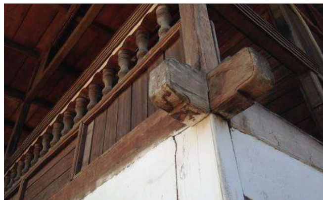
Figure 2. A sample of beam-column joint of traditional house in Manado (source: authors).
