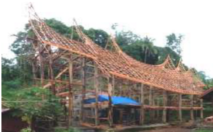
Figure 3. The Minangkabau Traditional Wooden House in West Sumatra, Indonesia (Pranata and Tobing, 2016)
