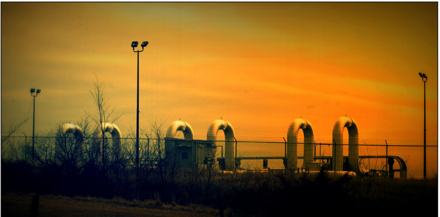
A pumping station on the Keystone pipeline, which transports Alberta tar sands oil to the United States.
