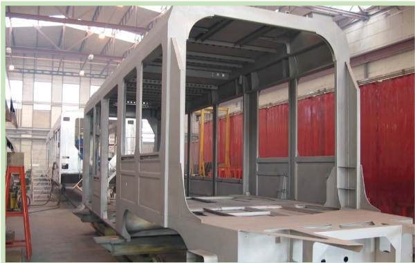
Fabrication of Tango light rail carriages in the workshop (Photo: ThyssenKrupp Nirosta)
