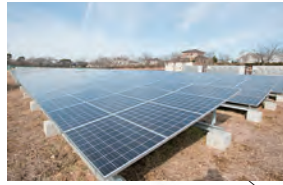
太陽光発電設備 Photovoltaic Facility
