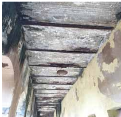
Deteriorated condition of the building ceiling
