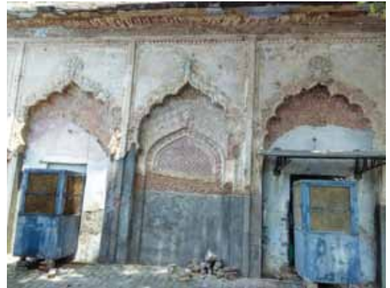
Detail of plaster loss and repairs with cement
