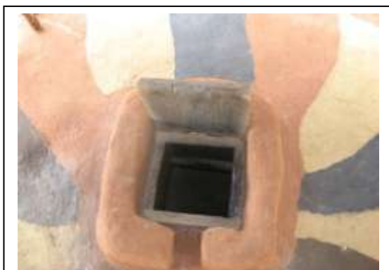
Protecting the well mouth in Kampampi, Nchelenge, with high lip, lid and apron. (Vertical view downwards)
