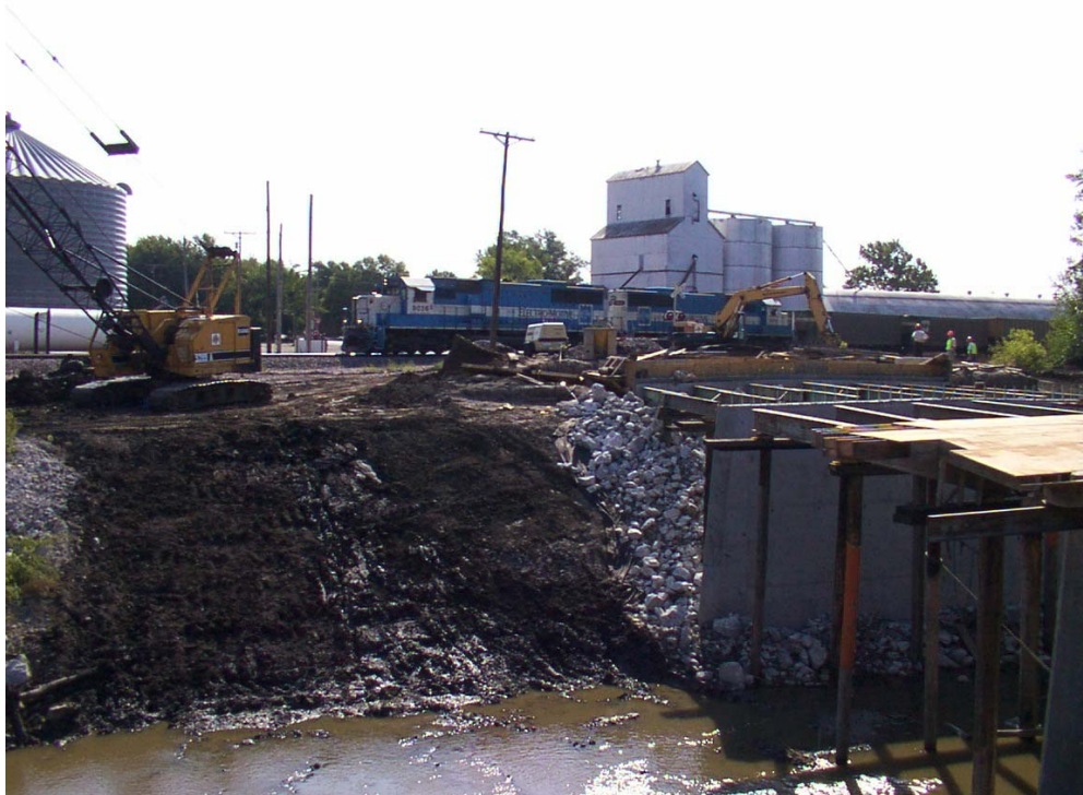
FIGURE 2 A railroad crossing is located immediately following the end of the bridge.
