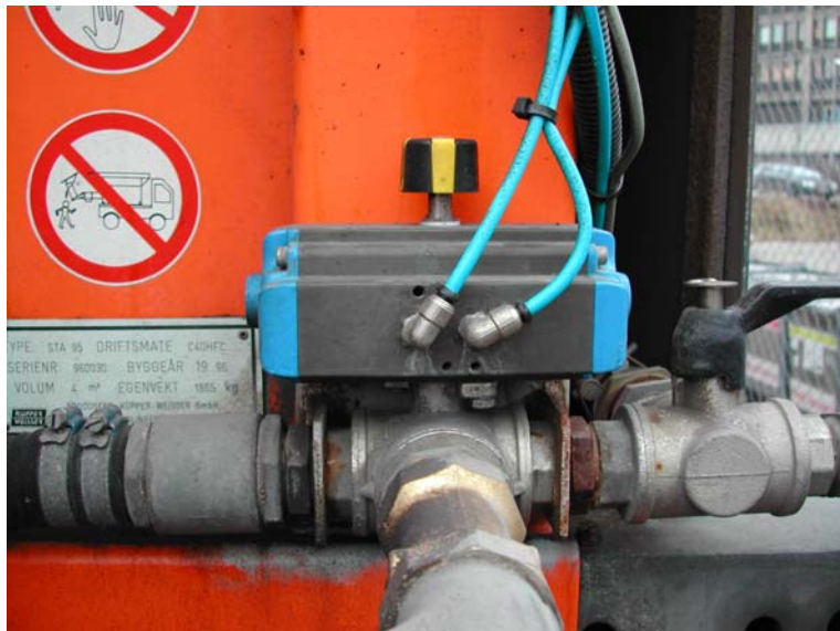
FIGURE 5 Valve system on the salt spreader in Oslo.
