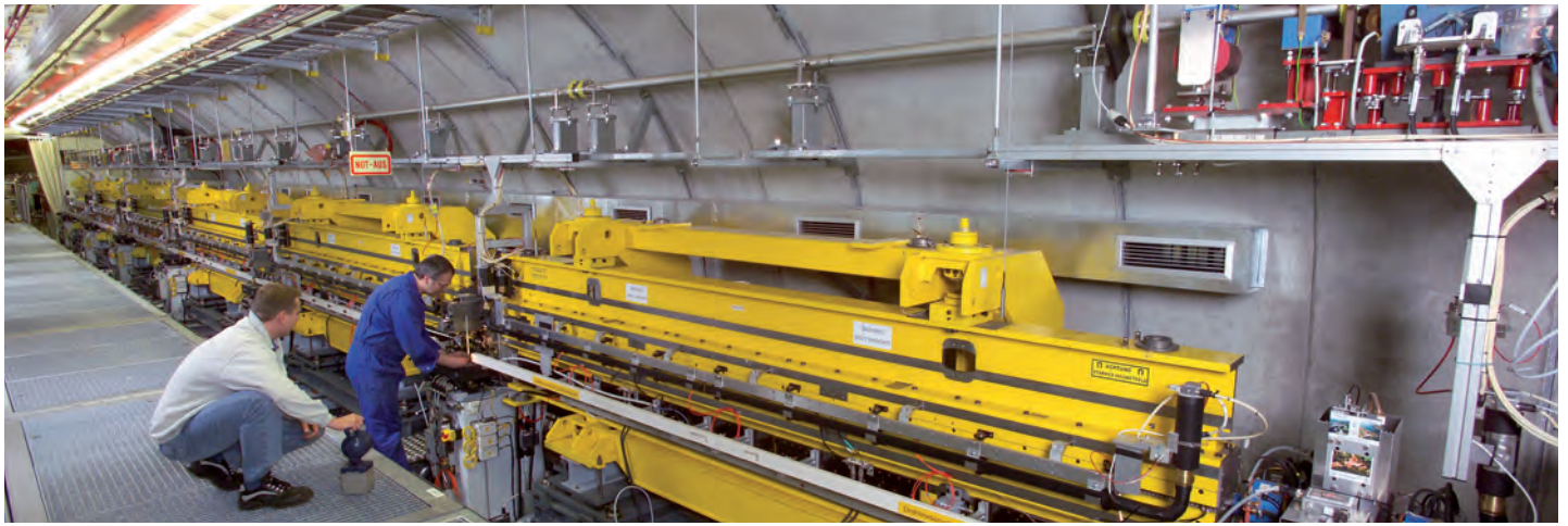
The undulator section in the FLASH tunnel
