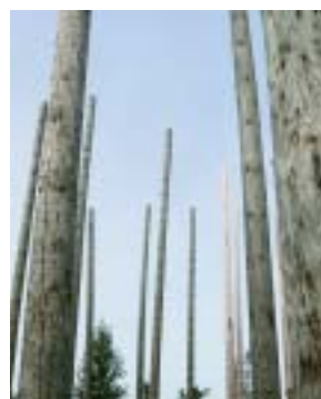
Poles treated with a new polymer additive.
