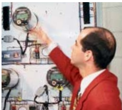
New electronic meters for business and large-power customers.
