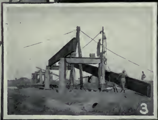
PROSPECTIVE AND COMPLETED ENGINEERING CONTRACTS BY A. J. CORBETT & CO. 1. PLAN OF THE MENAM BRIDGE, ROYAL STATE RAILWAYS. 2. THE ENGINE SHEDS OF THE ROYAL SIAMESE STATE RAILWAYS. 3. SEE YEK BRIDGE (in course of construction; 4 spans of 10 metres). (See p. 198.)
