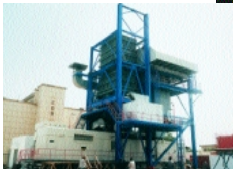
The 37.4-MW Bel-Air gas-turbine power plant in Senegal was built and commissioned in cooperation with a Québec company and a Senegalese partner.
